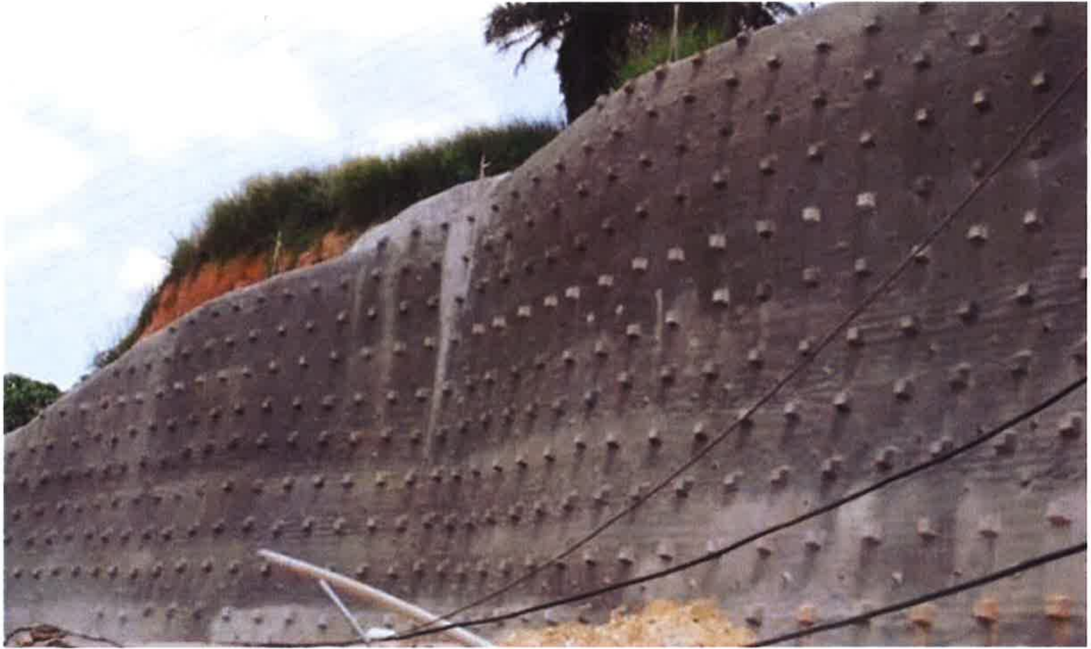
↑ Soil nail wall w/ no veneer
