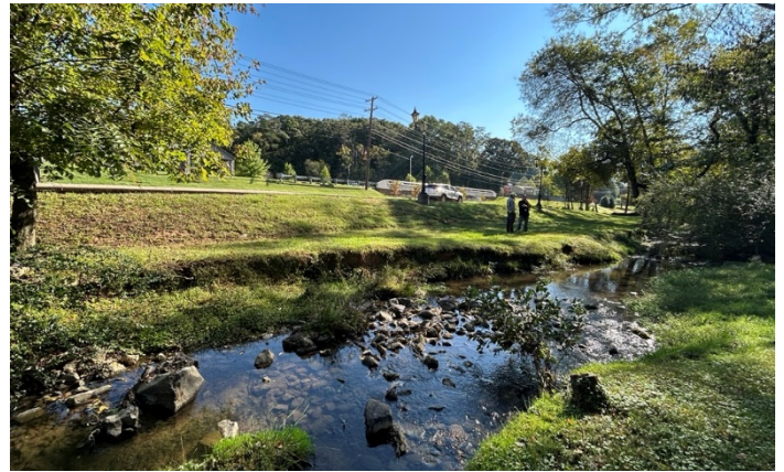
Project Site October 2025- bank slumping shows continued erosion
