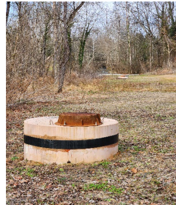
FUD sanitary sewer main
